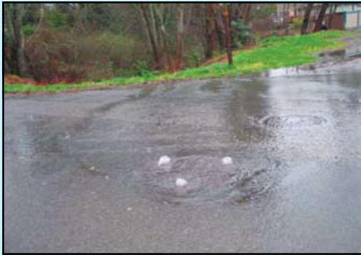
Using drains and toilets as trash cans may create sewer overflows into streets and water bodies.
